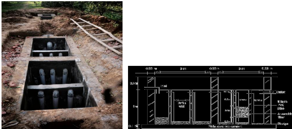
Figure 13 : Improvised Septic Tank
