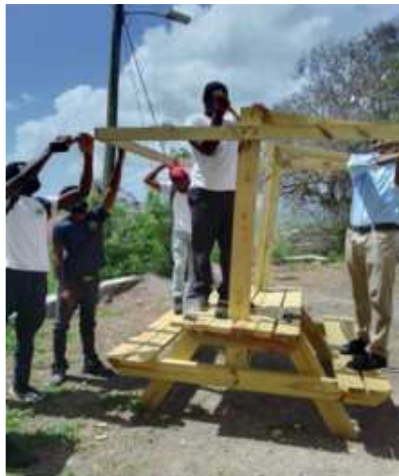
Students of the Industrial Technology Department building benches at Antigua State College
