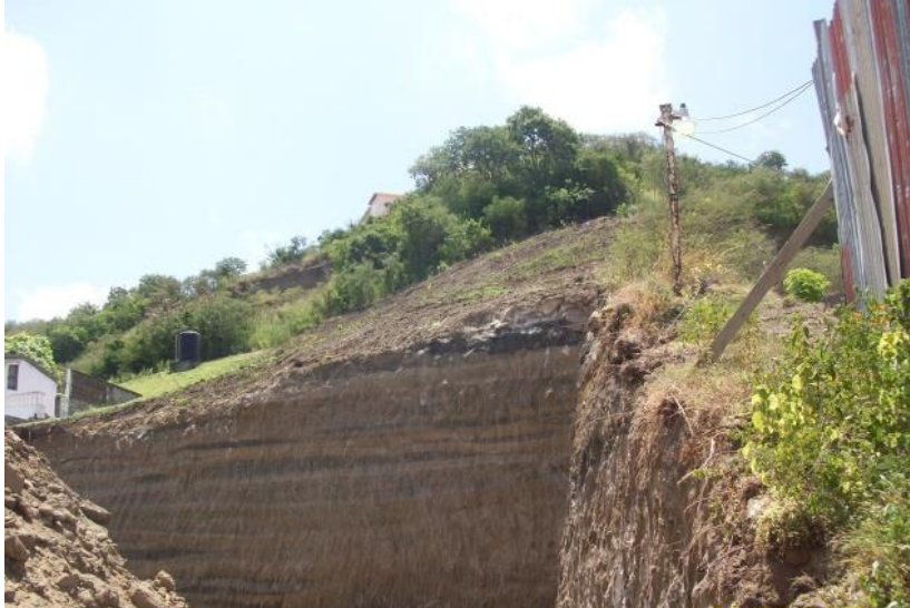
Photo Plate 1.1.2.1-2: Land excavated at very steep slopes, Southern Grenada
