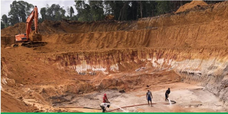
1) Excavator clears vegetation, opens pit and piles material for processing 2) 4-8" suction pumps with 2-4" spurting hoses (jets) create slurry from open pit face or piled material
