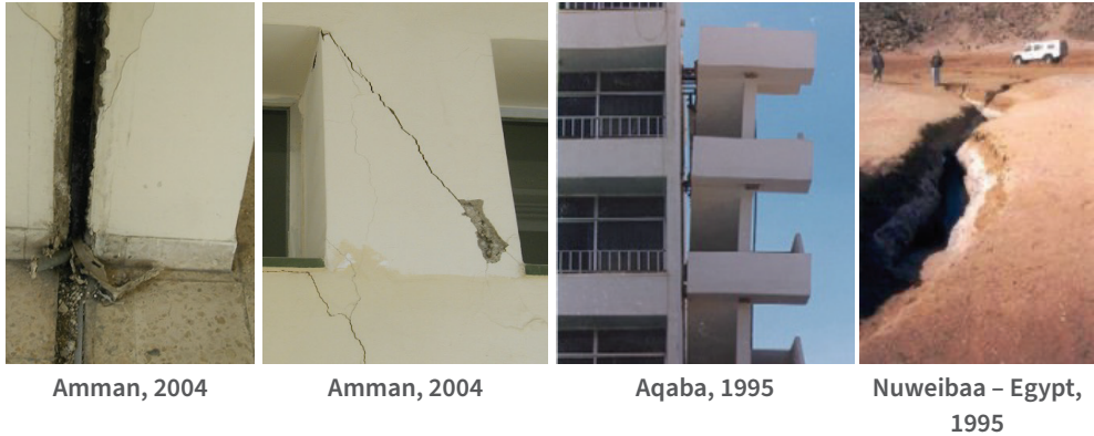
Figure 5: Selected picture for the damage caused by the earthquakes of 1995 & 2004 ▲
