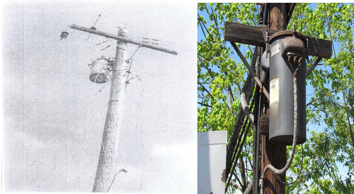
Figure 9. Type of transformers used before 1989. Pole mounted transformer made in Germany
