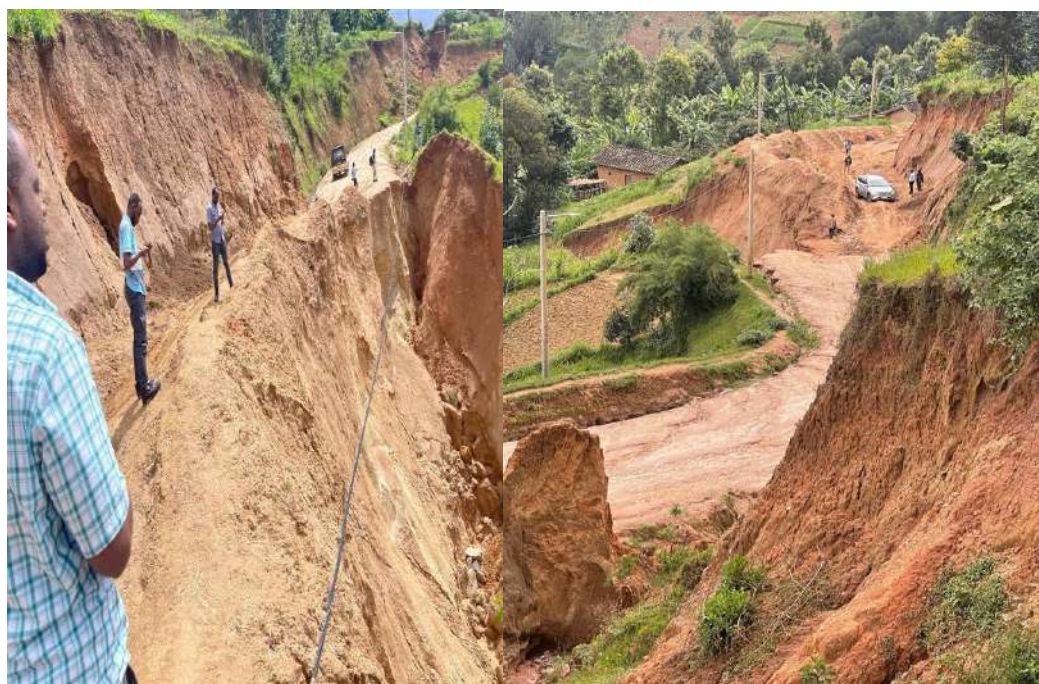
Figure 25: In Nyabimata sector, the improper Road drainage caused the landslide and road deterioration
