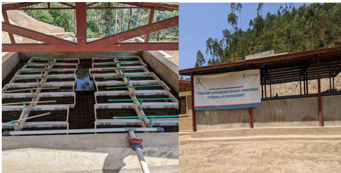
Figure 48. Wastewater treatment plant in Base Sector
