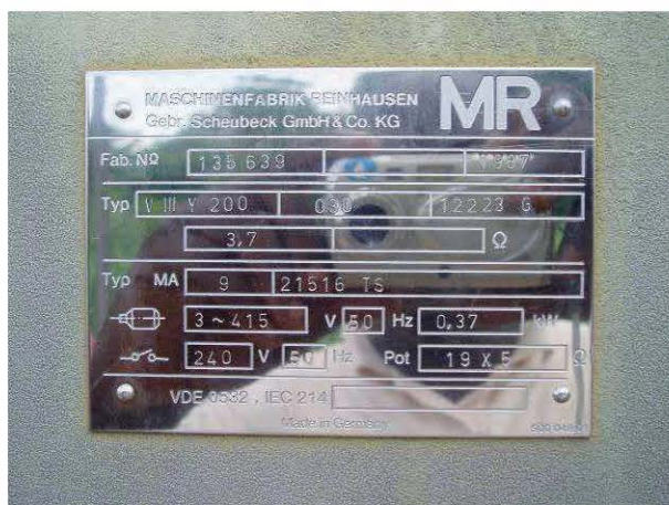
Figure 7: Transformer name plate in Bo-Kenema
