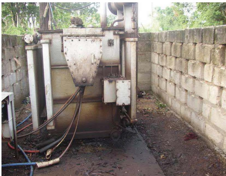
Figure 6: Oil spillage at the BKPS Kenema reservation sub-station
