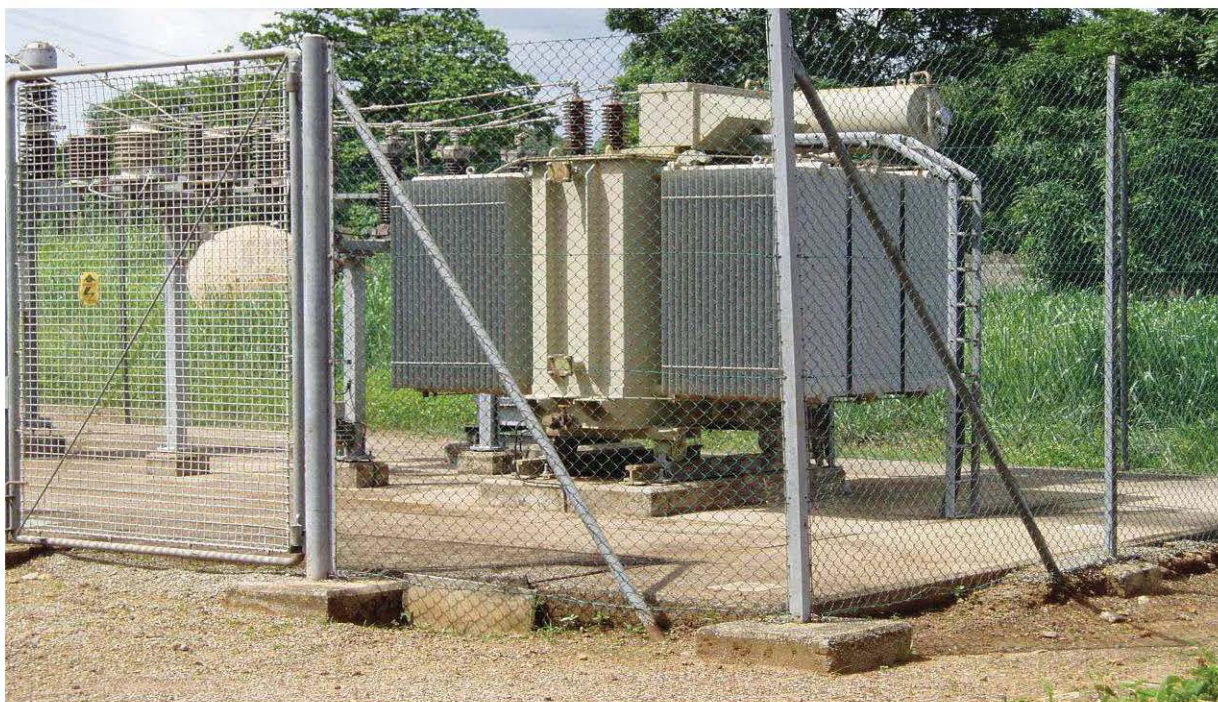
Figure 5: Main transformer receiving current from source - Bo
