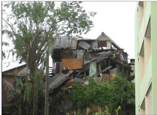
Figure 2: Damage caused by Hurricane Dean, 2007
