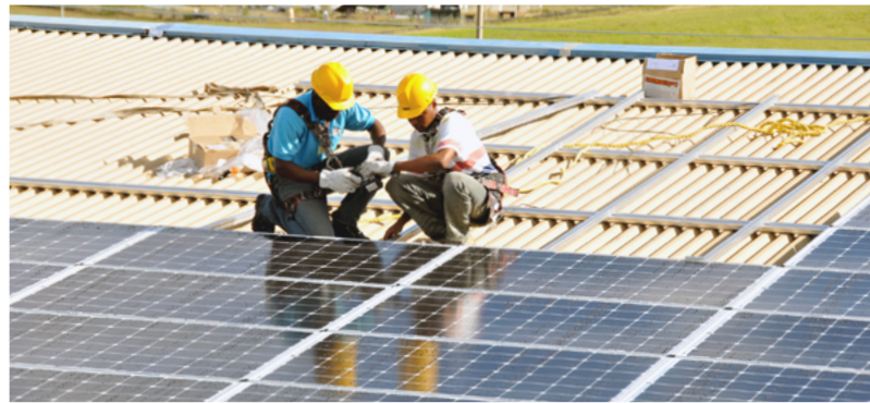
Photo: St. Lucia Electricity Services, Limited
