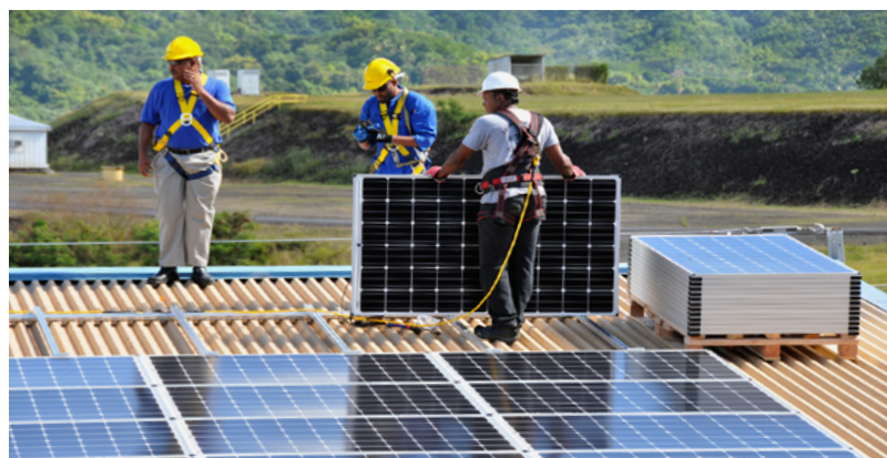
Photo: St. Lucia Electricity Services, Limited
