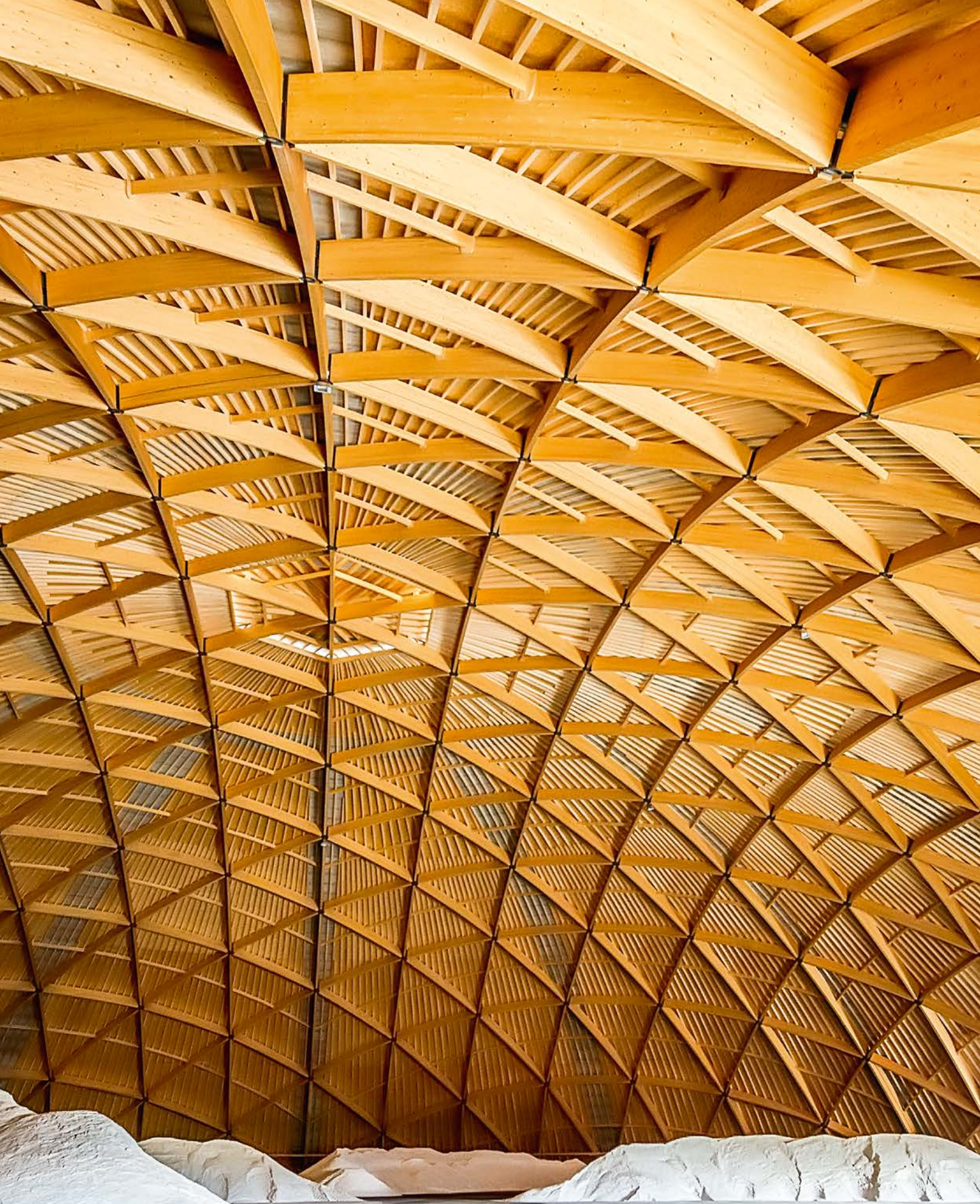
Timber dome of the Riburg salt works (Aargau): this timber dome, the largest of its kind in Europe, showcases the innovative strength of Switzerland's timber sector.
