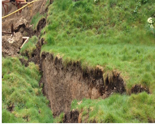
Bad practice in earthworks which may cause erosion during construction improper earthworks which may cause erosion during construction
