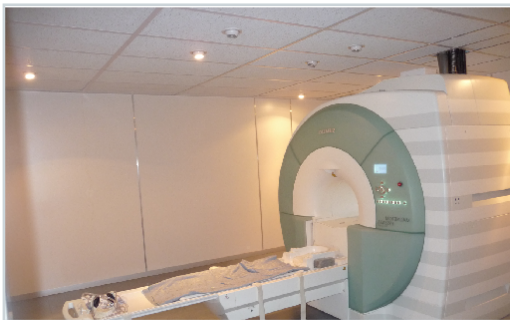
MRI equipment at Cancer Hospital
