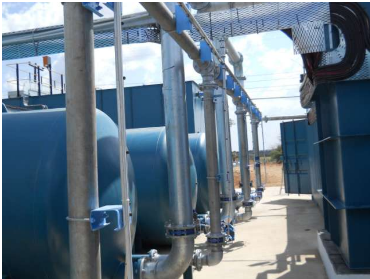
Typical Water Supply Development – Contracted Chongwe Water Treatment Plant, Lusaka Water
