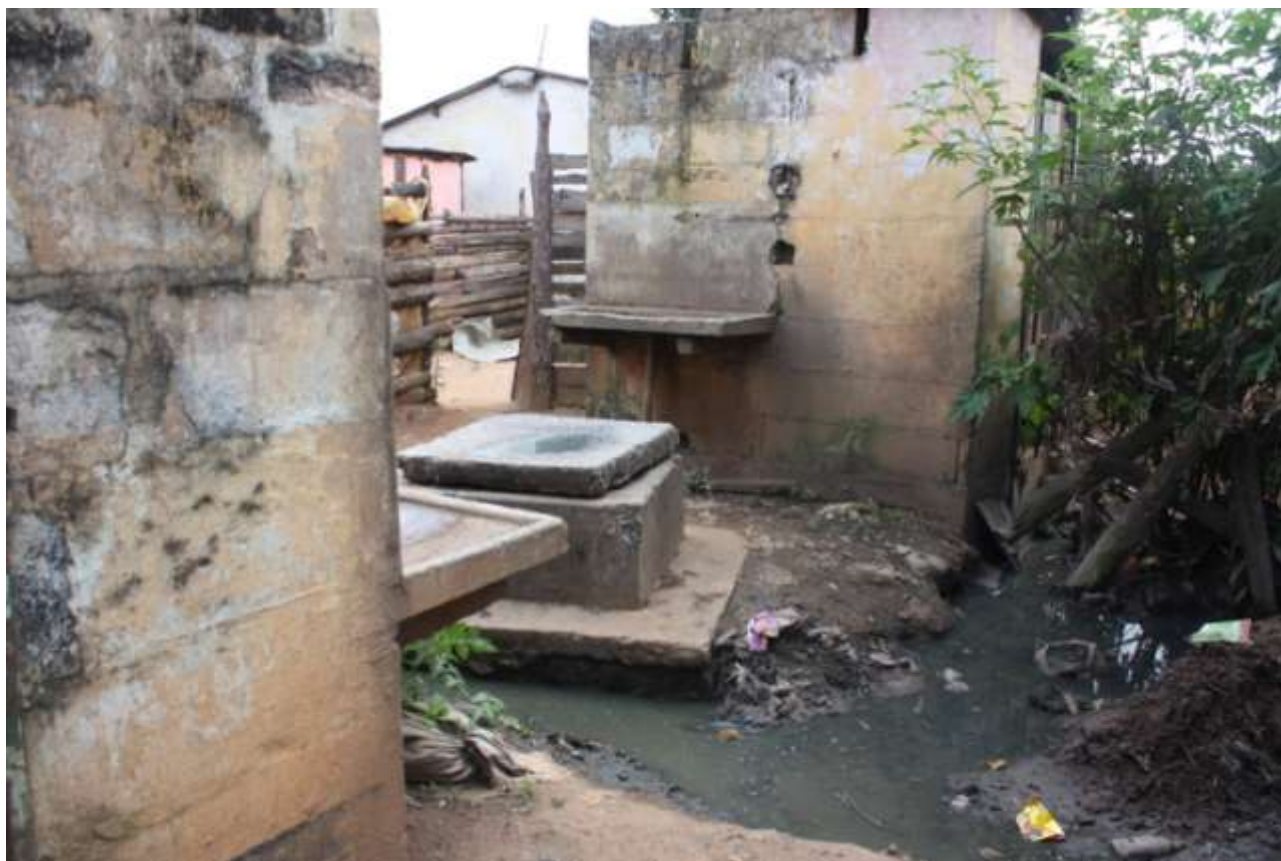
Dilapidated Infrastructure resulting in reduced access to water supply and sanitation services
