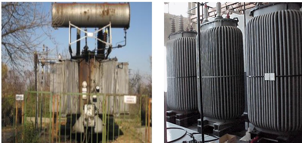
Image 1: PCB-containing transformers in use, also operated in Bulgaria
