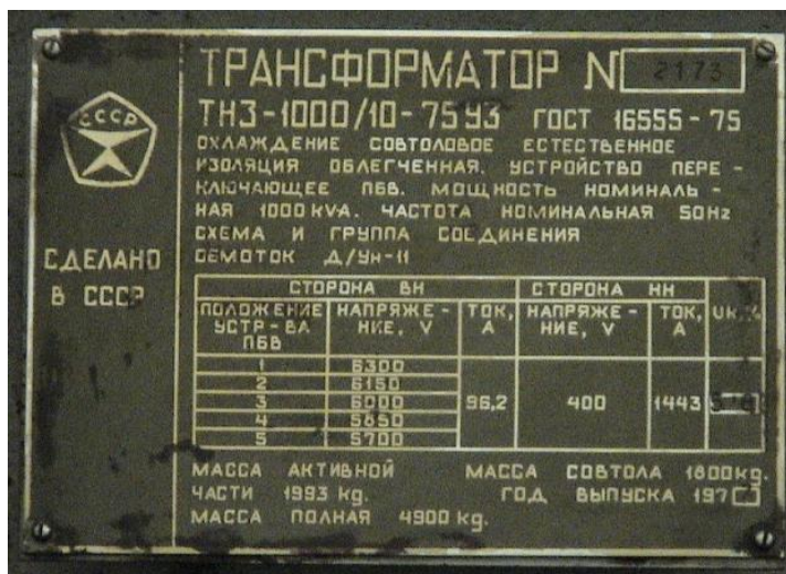
Image 2: Manufacturer sign of a Russian PCB transformer (Sovtol), operated in Bulgaria
