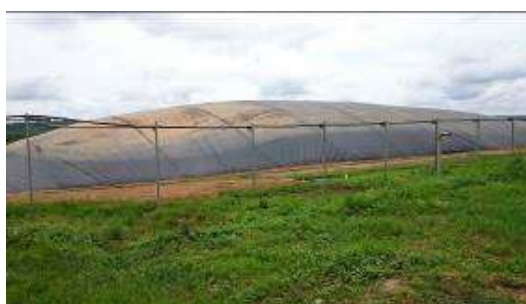
1000m 3 biogas reactor
