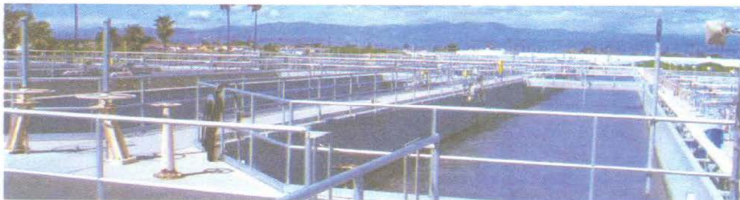
Loji pengolahan air sisa. Wastewater treatment plant.
