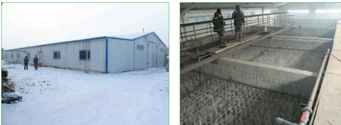
Figure 68. Newly established wastewater pre-treatment plant of Arildii LLC
