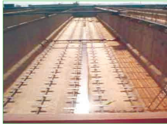
Aeration tank diffuser
