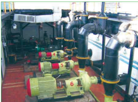
Return sludge pump
