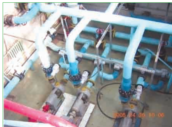
Pump station for raw residue
