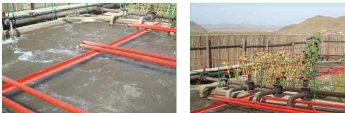
Figure 65. Bio factory WWTP clarifiers
