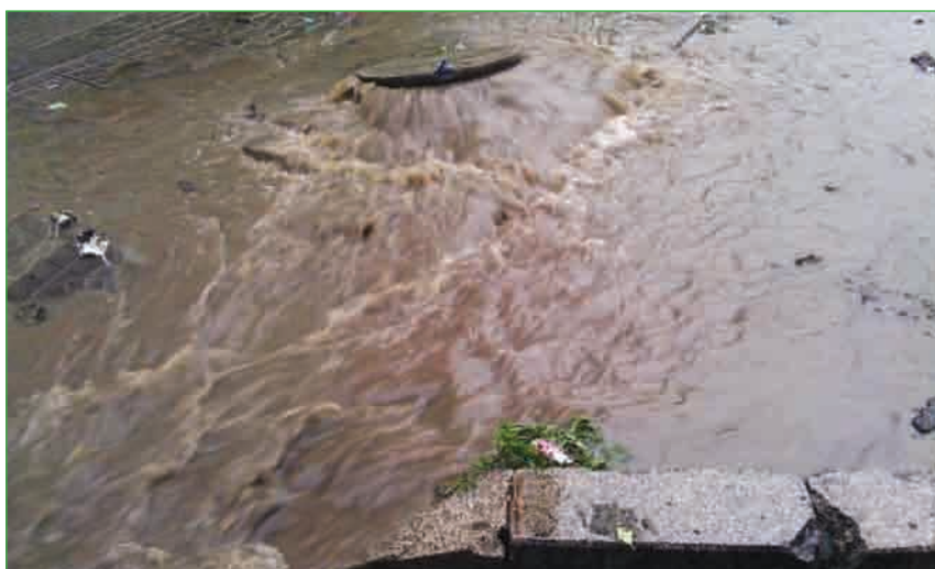
Figure 72. Clogging of rain water drainage pipeline during the flood
