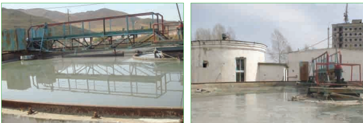
Figure 66. Khargia industrial wastewater pre-treatment plant
