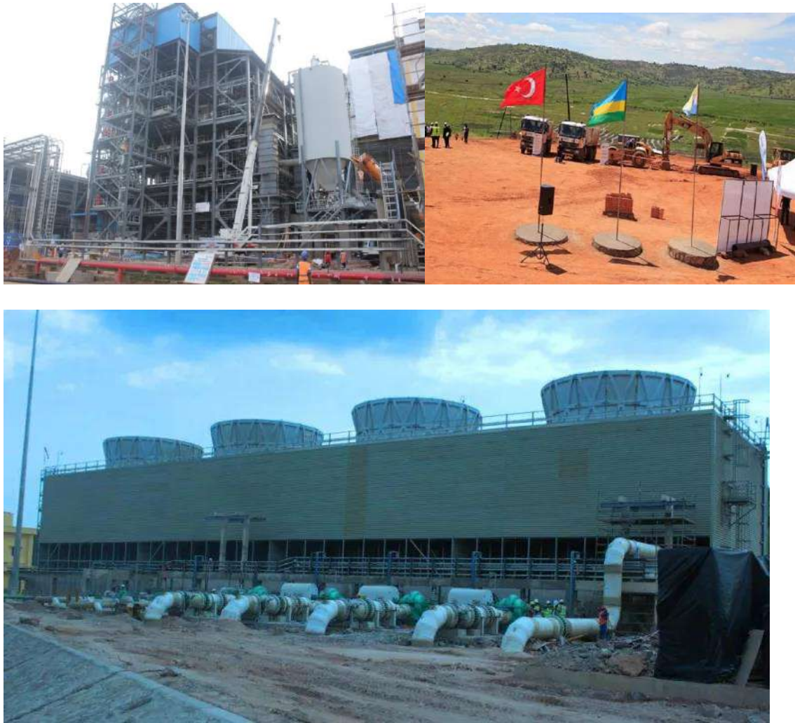
Figure 22: Peat Power plant in Gisagara District
