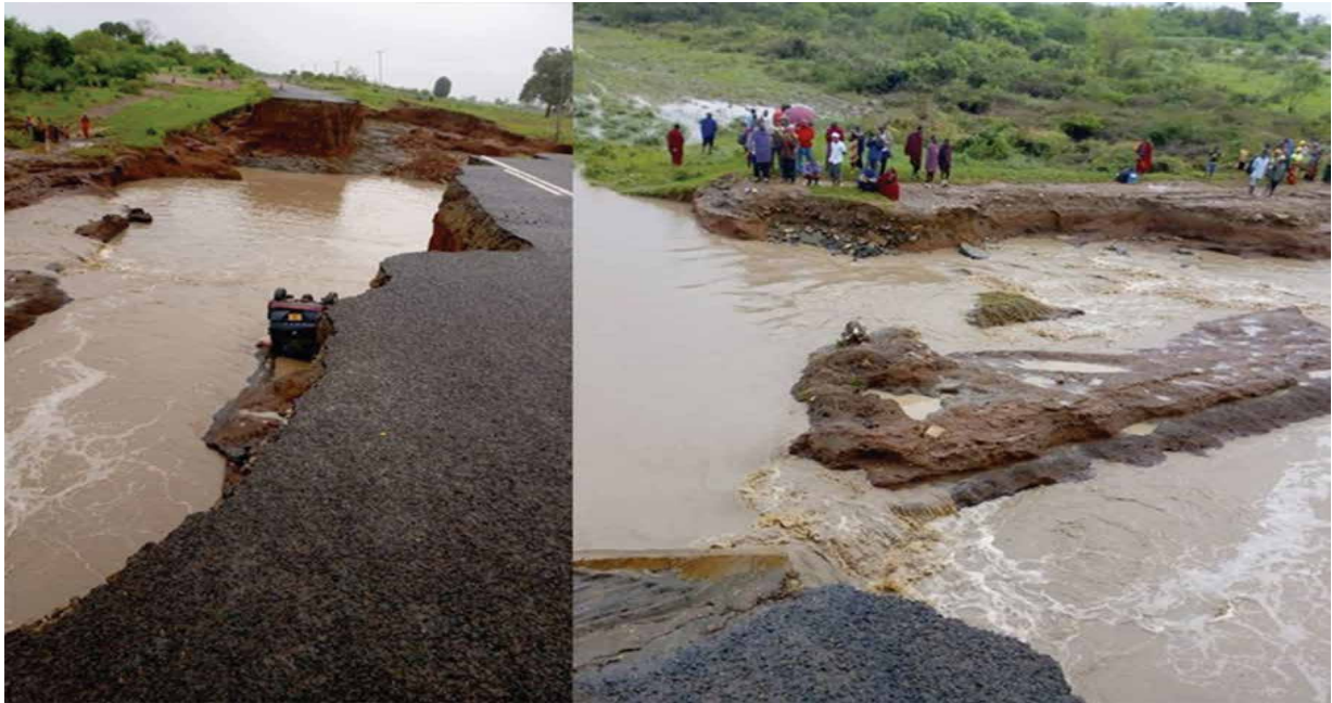
Photo 5: Effects of floods on road infrastructures in Handeni, Tanga Region
